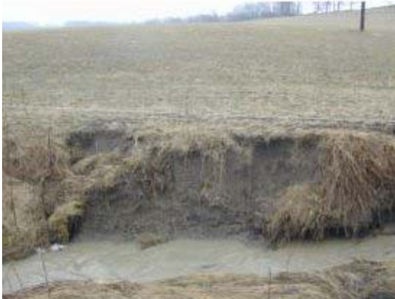
Figure 2.5 Bank erosion in close proximity to cultivation (Photograph by L. Øygarden.)
