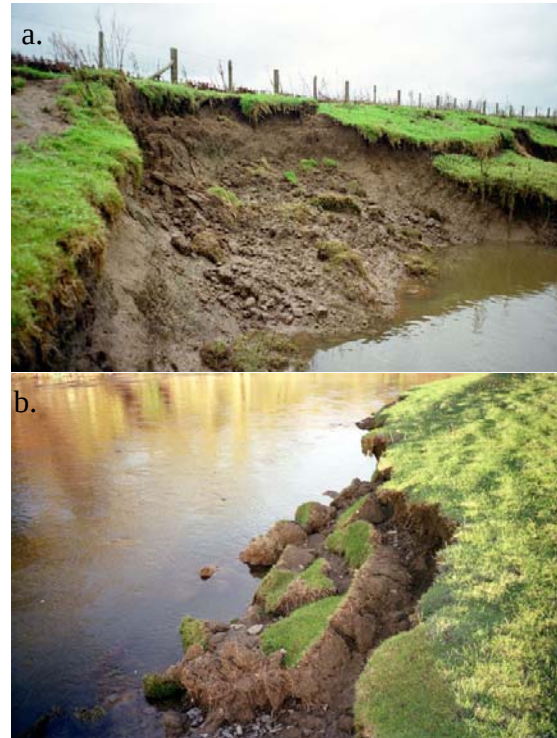
Figure 2.6 Bank erosion (a, b) R Swale, northern England UK (Photographs by P N Owens)
